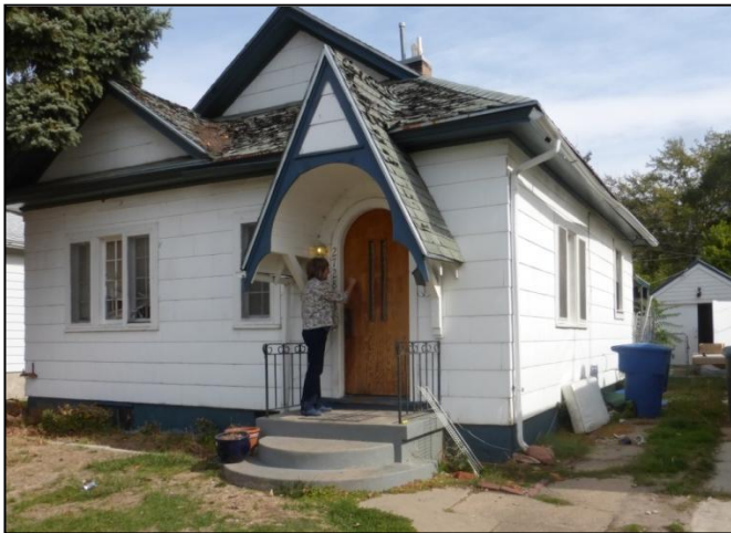
The house as it looked during our visit in October of 2014. Notice the cracked driveway, the rotting roof and the garbage strewn about.
